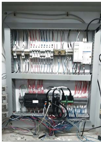
Figure 2: A new control system for the jaw crusher was built around the AutomationDirect BRX PLC, a versatile stackable micro brick platform with I/O expansion modules. Because the existing field wires were too short, a preconfigured ZIPLink cabling system was used to facilitate connections.
