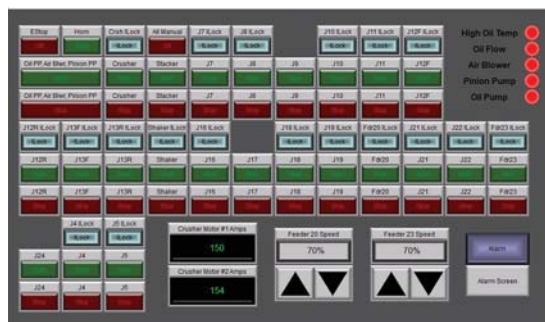
Figure 3: The primary user interface for the jaw crusher is built on the AutomationDirect C-more CM5 series 12 in. color touchscreen HMI. With space to display all the jaw crusher and feeder settings, the number of screens to navigate was reduced allowing operators to quickly confirm status at a glance.
