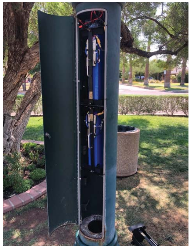
Solar energy storage installation site at South Mountain Park, City of Phoenix.
