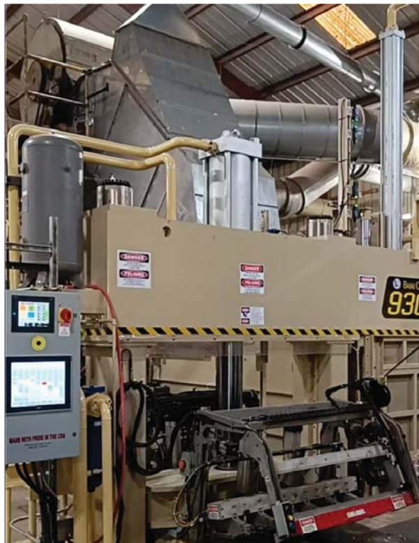
3. The cotton press, with the touchscreen human machine interface (HMI) shown at left. The Productivity PLC from AutomationDirect integrates well with AutomationDirect C-More HMIs, as well as similar products from other manufacturers (shown).
