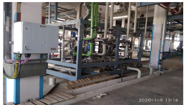
Figure 2: Field junction boxes are located near the sensors and actuators wired to them.
