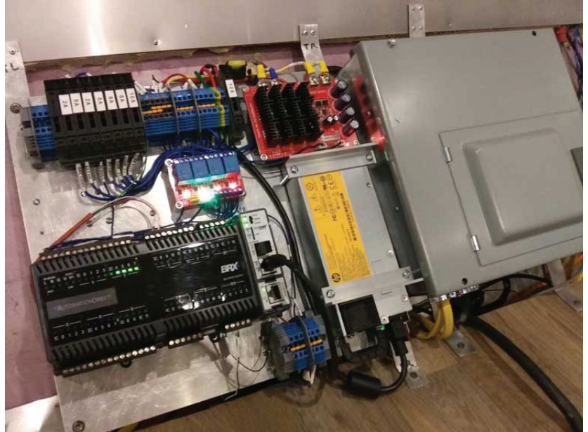
An AutomationDirect BRX PLC orchestrates all camper monitoring and control functionality, and it interfaces with the electrical systems using sensors and solid-state relays.
