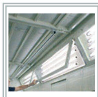
Eight 4-Tube LED light fixtures with hinged access for ease of cleaning and maintenance.
