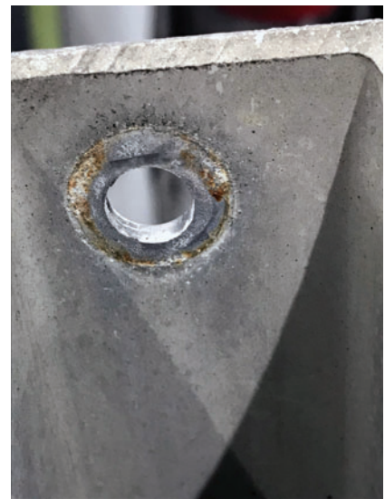
CORROSION EVIDENT after the fastener was removed. Galvanic corrosion can form between the two different metal surfaces.
