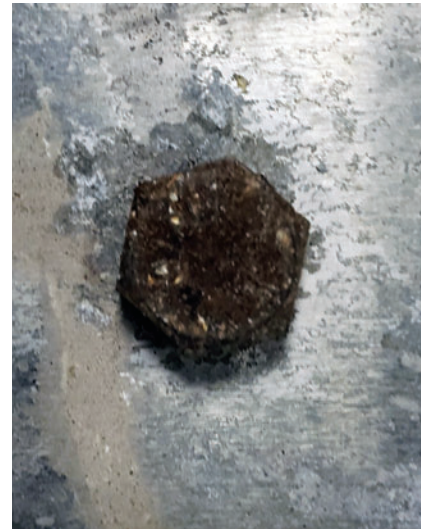
GALVANIC CORROSION formed due to using a steel fastener with an aluminum panel.
