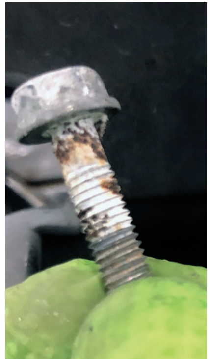
GALVANIC CORROSION can form on the threads of a screw, nut or bolt before being noticeable in use.
