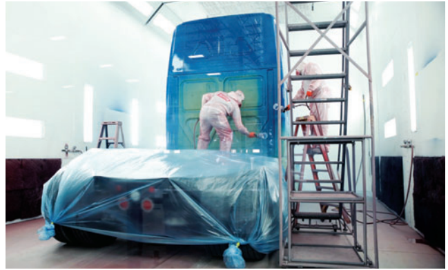
KEYSTONE SUPPLIES the Axalta Coating Systems Imron paint, sprayed in Uni-Cure booths.
